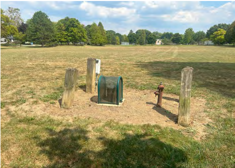
On Site Well West of Soccer Fields
