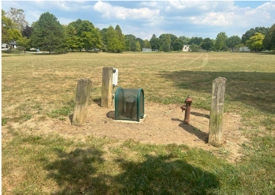
On Site Well West of Soccer Fields
